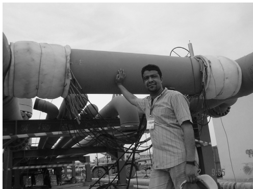
Figure 1.b. Gas pipeline in compression system
