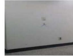
No fire extinguishers
