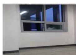
Abnormal: the window is opened
