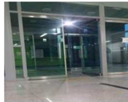
Abnormal: the door is open
